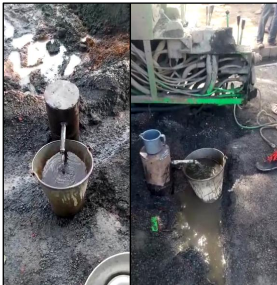
Fig. 3.1 Autoflow Well at Washim District, Maharashtra
